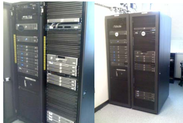
Figure 4, Valador maintains secure servers for several Government customers in our temperature controlled server room.
